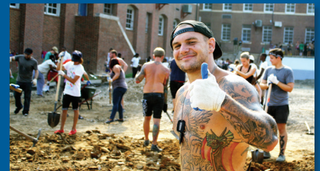
Volunteers from the Vans Warped Tour pitch in to remove asphalt at a school in Baltimore's Hampden neighborhood. Photo credit: Blue Water Baltimore.
